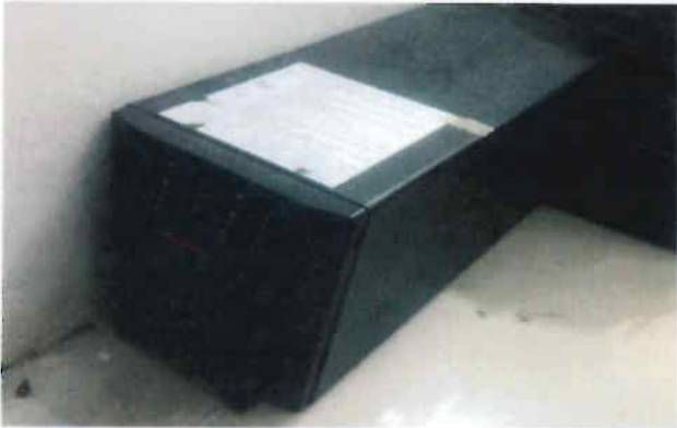
Small UPS - Faulty
