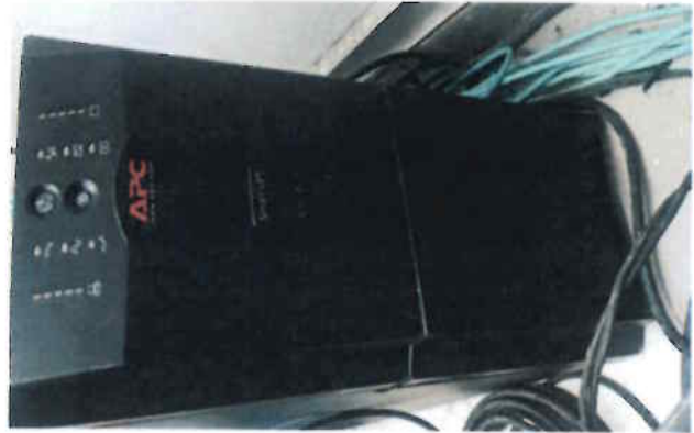
Large UPS - Faulty
