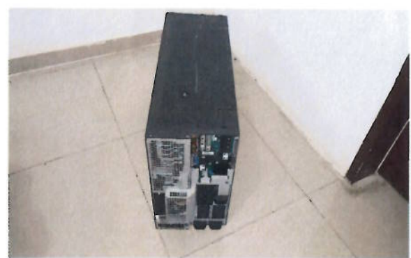
Large UPS - Faulty
