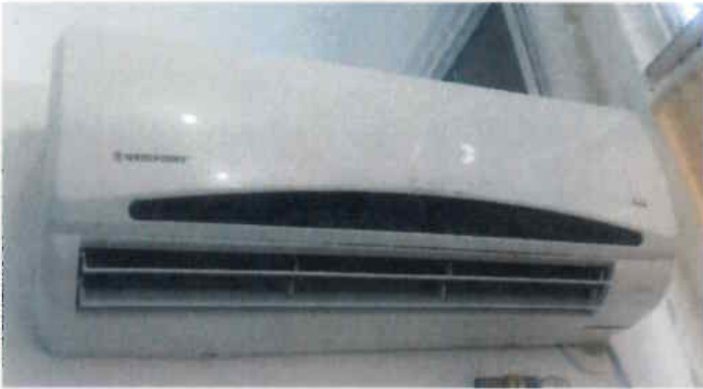
Wall mounted AC's (Multiple brands) - 17 pcs
