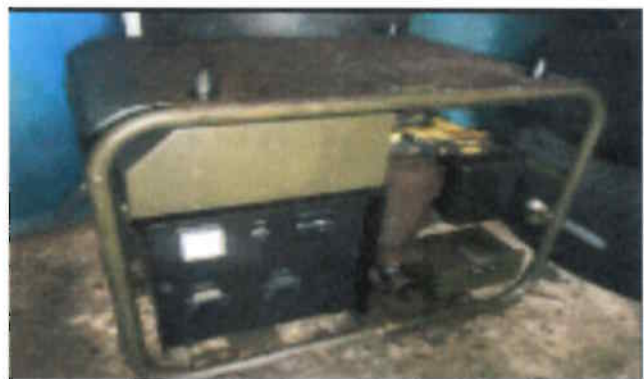
2.5 Kva generator - Rusty all over
