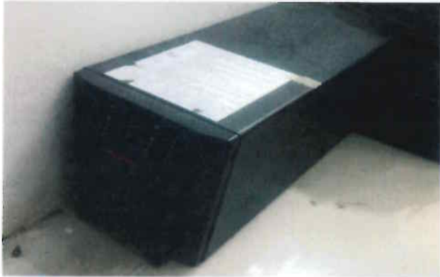
Small UPS - Faulty
