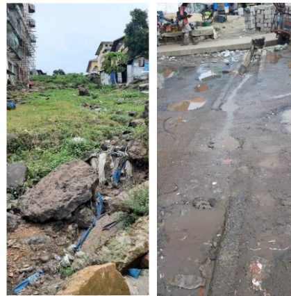
Photo 2: Open Space between Water Street and Front Street (left), Photo 3: Clogged drain at Water Street towards Mesurado Estuary (right)
